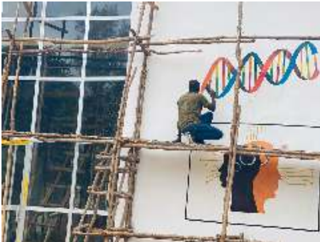
Drawing DNA on the STEM and Biomedical Center Under Construction, Kenema Sierra Leone, West Africa
